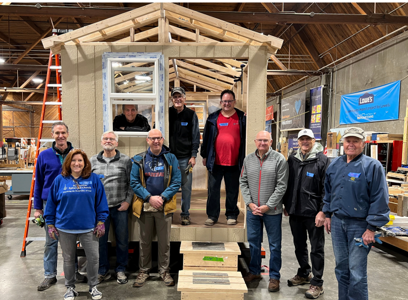
St. Thomas Members constructing a Tiny Home at Sound Foundations of Seattle this week.
